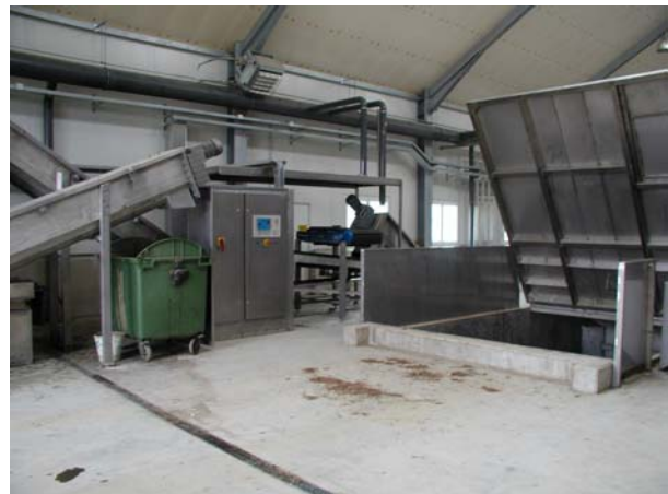
Biogas Plant Hartberg-Habersdorf © LEA
